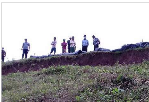
Figure 6-43: Slip section of Bandaraulpotha Tank Bund in Padaviya Division on 20.12.2021
