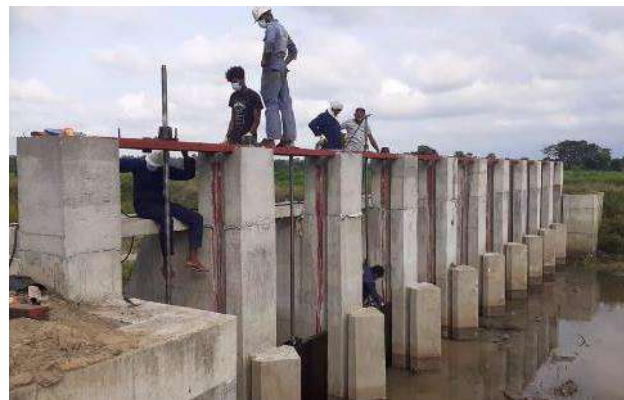
Figure 8-12: Fabrication and Installation of 40 Nos anicut gates and Hoisting mechanism in Batticloa Range
