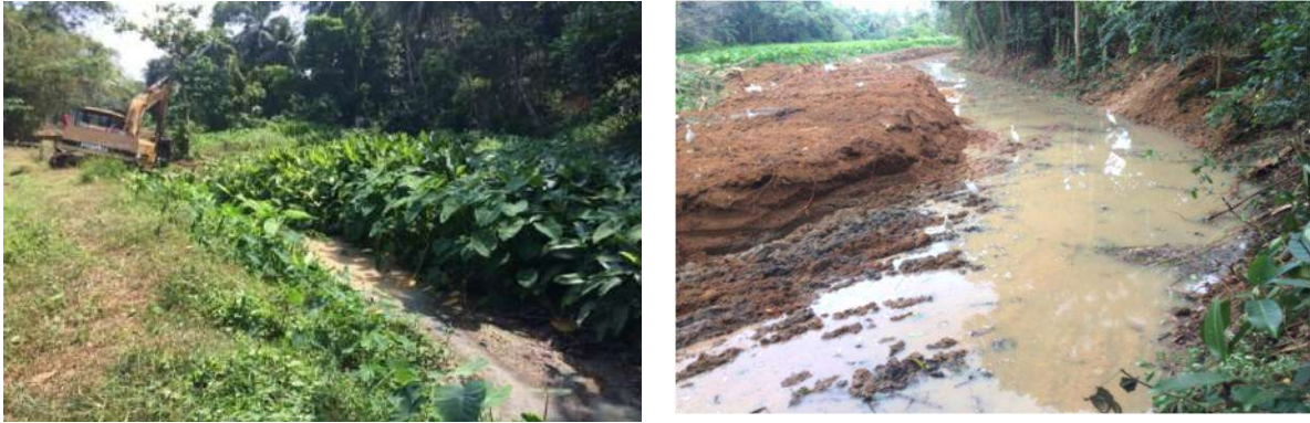
Figure 7-13: Removing plants & obstacles in Samadara ela drainage canal 3rd section in Makandura scheme
