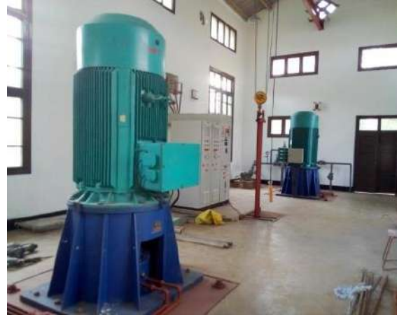
Figure 7-23: Hammaliya Pump House
