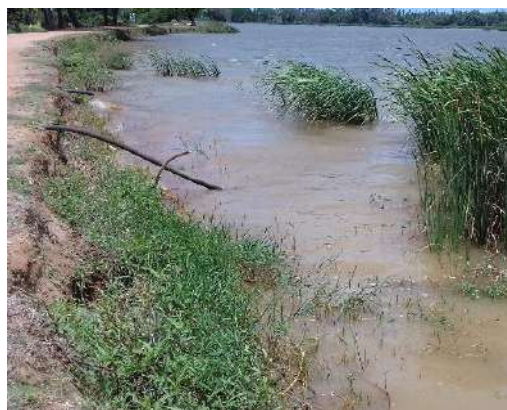
Figure 6-44: Upstream bund erosion in Debarawewa Tank Bund in Tissamaharama Division on 27.07.2021
