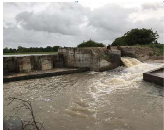
Figure 6-37: Construction of emergency spill at Kompansaithan feeder tank in irattaikulam main canal in Giants Tank scheme
