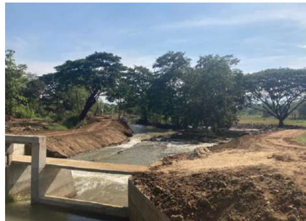
Figure 5-11: Thissapura Tank Spill tail canal
