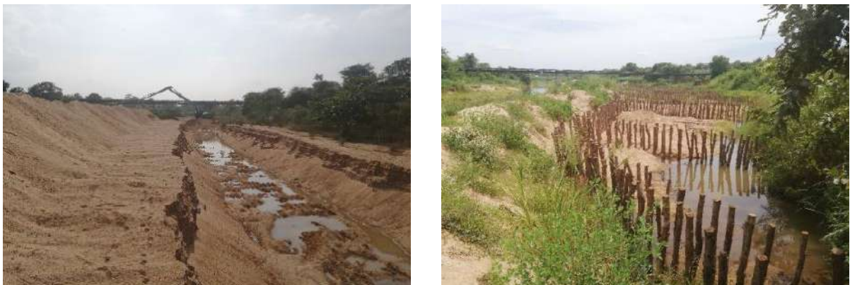
Figure 7-7: Construction of timber pile in RB Embankment of Gal oya River near sugar factory
