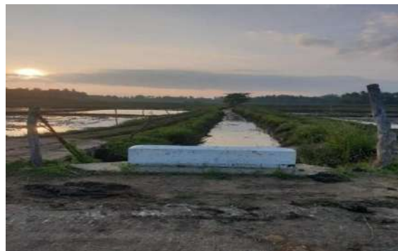
Figure 5-42: Construction of 16m conduit at the end of Humbaskumbura gate HLMC Yodhawewa scheme
