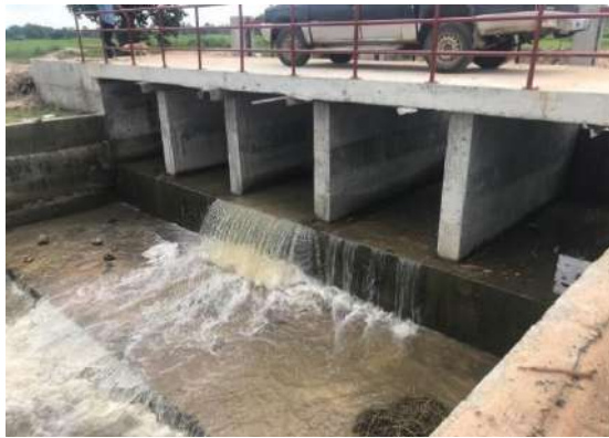
Figure 6-40: Reconstruction of drainage outlet cum bridge at stn.13+942 in RB main channel in Unnichchai scheme
