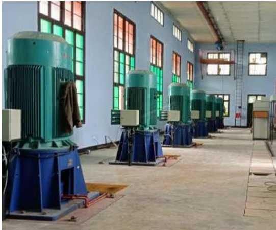
Figure 7-22: Divithura Pump House
