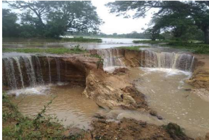
Figure 12-8: Scoured Section of Katagamuwa Spillway
