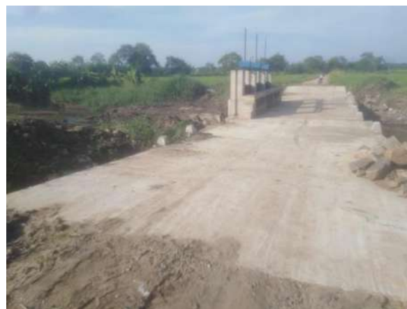
Figure 11-151: Construction of 3 bay regulators across the Woulbokkuwa drainage canal in Kaudulla Division
