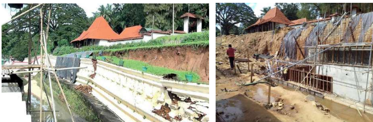
Figure 12-7: Collapsed retaining wall and constructions of RW at Sri Dalada Maligawa
