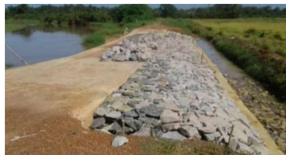
Figure 11-60: Boulder packing of U/S of causeway at 1+650 at Bogahapitiya anicut in Welikada scheme
