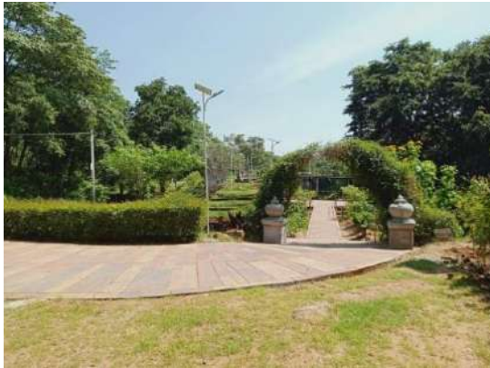
Figure 11-165: Installing Solar lights, CCTV camera system & Improvements the appearance in Elahera main Anicut
