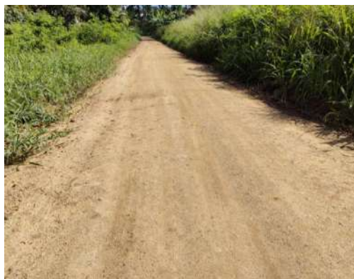
Figure 11-159: Improvements to D01 canal Bund from 0+000 to 4+100 in Samagi DCO Area in Kaudulla Division
