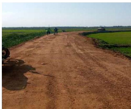
Figure 11-7: Improvements to Kiramakkuddy Road stn. From 0+000 to 2+000 in Block 'J' Scheme, Sammanthurai Division
