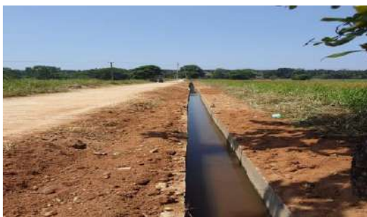
Figure 11-59: Concrete Canal lining for first branch of RBMC from 0+200 to 0+367 – Idallawala Scheme
