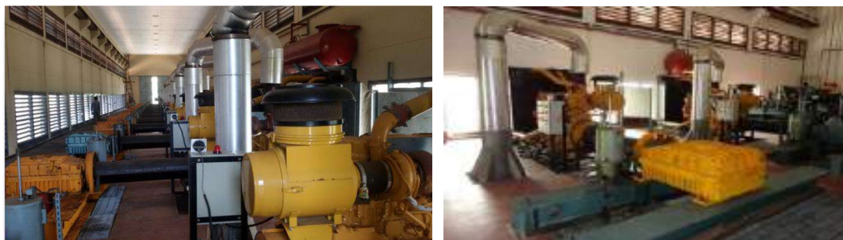
Figure 7-17: Improvement Works of Magallagoda, Thalgahagoda Pump Houses
