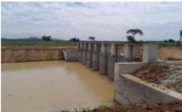
Figure 11-73: Improvement to Pilayarady Anicut/Regulator in Kalvankai River, Rugam Scheme
